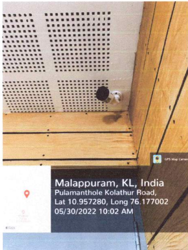
LECTURE HALL CCTV
